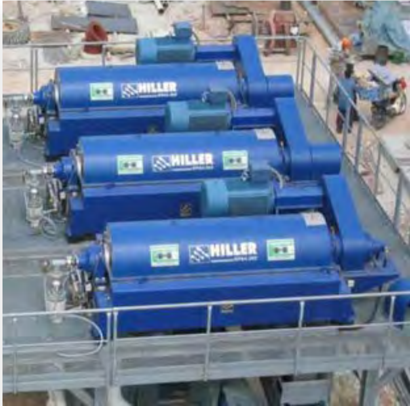
Centrifuge dewatering equipment
